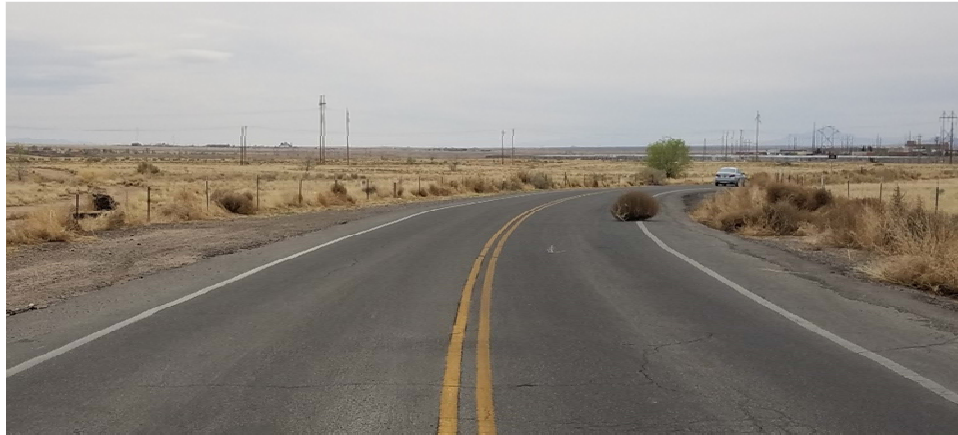
FIGURE IIIB.2. INNOVATION PKY. FROM SOUTH OF RESEARCH RD. TO IPOC EAST DRIVEWAY TYPICAL SECTION
